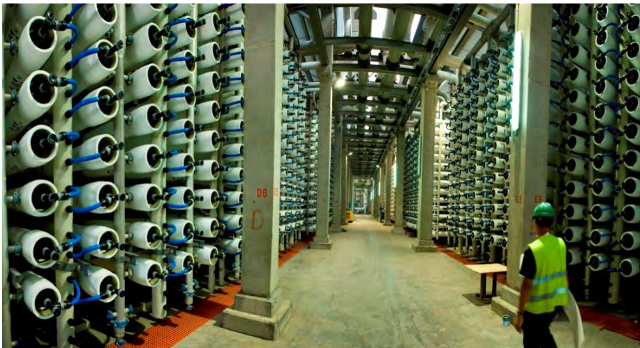
Figure 5.3 photo of the Hadera SWRO plant ( www.ide-tech.com )
